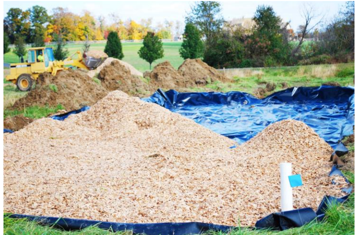
(Above) This is a bioreactor under construction on Fair Hill Farm, Kent County, MD. The pit is being filled with woodchips.
